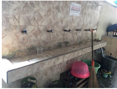
Gambar 7. Kran Distribusi Air Minum
