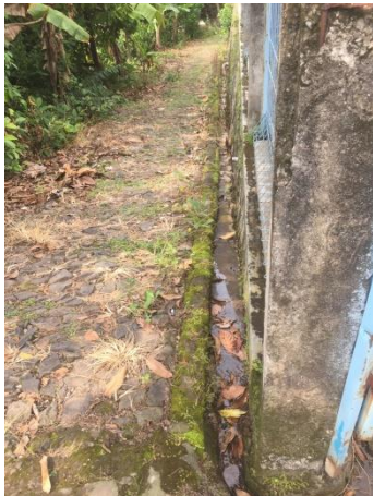
Kondisi Saluran Air DAMIU Made
