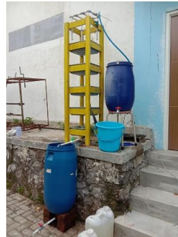
Gambar 10. Penataan Multiple Tray Aerator dan bak adsorpsi
